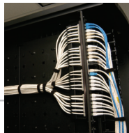
End-of-Row Vertical Patch Panels
