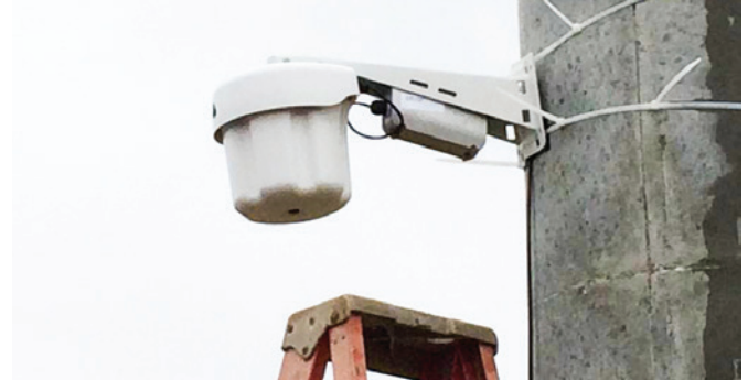
PoE extender pictured with Aruba AP275 Wi-Fi access point
