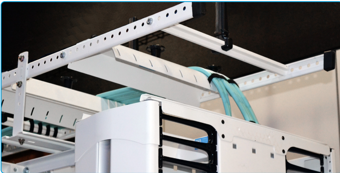
Figure 1: Advancements in cable pathway include cable runway (ladder rack) with adjustable cross members to quickly and easily correct alignment issues and tool-less pathway accessories to separate, guide and support cables. Photo shows CPI Adjustable Cable Runway, Tool-Less Radius Drop.
